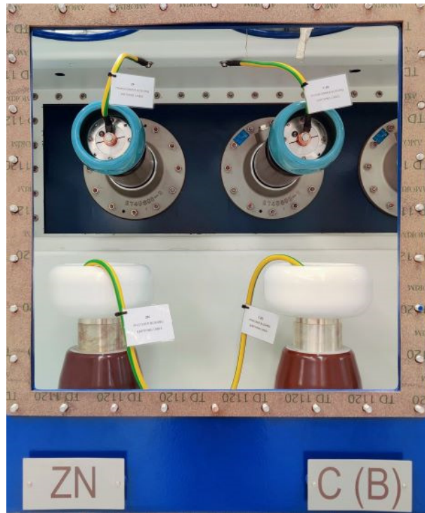
Internal View of Disconnection Chamber with all earth links in place
